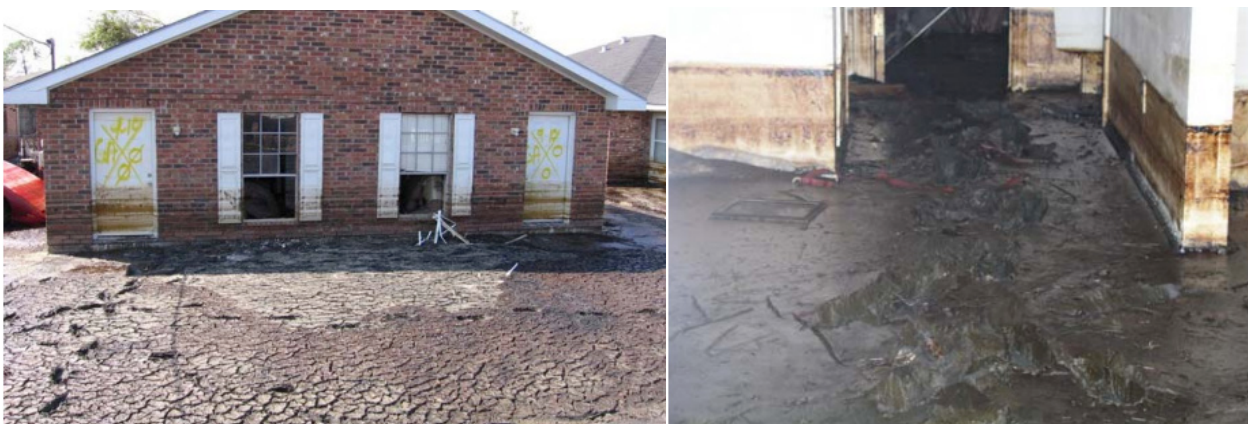
Crude oil deposits in and around homes following the Murphy Oil Spill in St. Bernard Parish, Louisiana.
