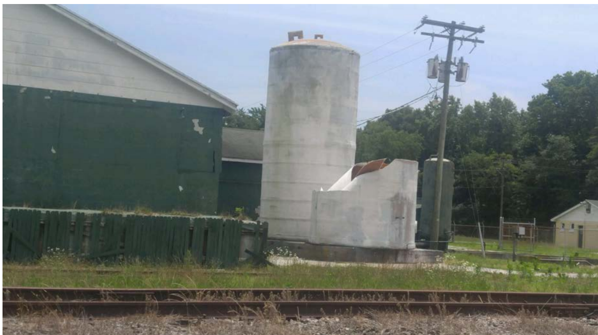
Derelict chemical storage tanks at a former agricultural supply depot in Savage Town, Accomack County, Virginia.
